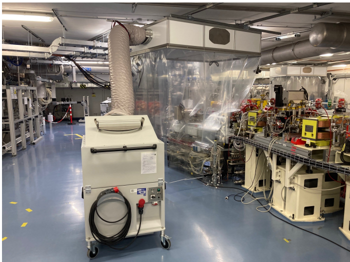
Rail system at ceiling to allow ISO5 flow-boxes everywhere at the machine to avoid particulates
